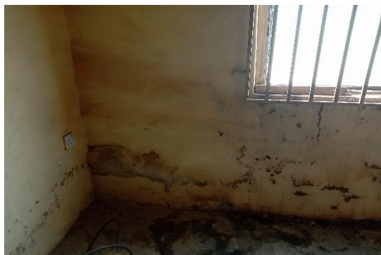
a) Peeling of paints
