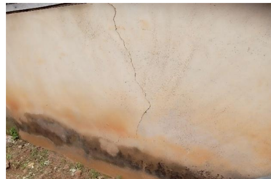
b) Dampness shown marks on basements
