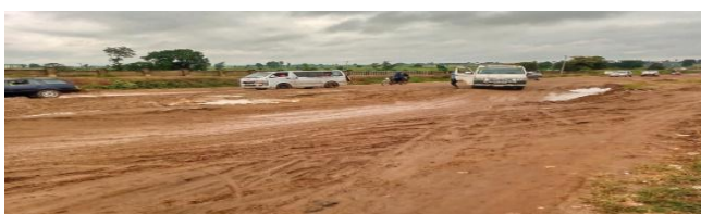
Unpaved road condition (Nasarawa urban area)
